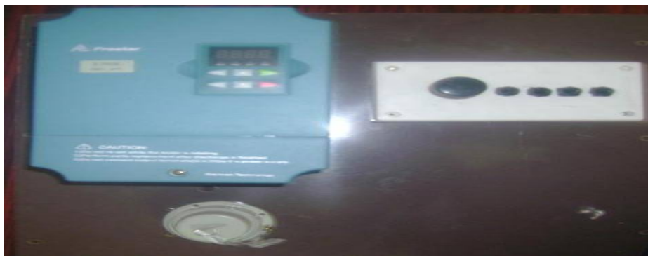
Fig 6: Variable Frequency Drive with its circuit board.
